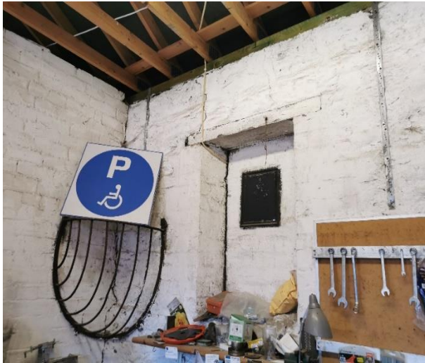
Photograph 9: Coach house internal wall separating from outer walls
