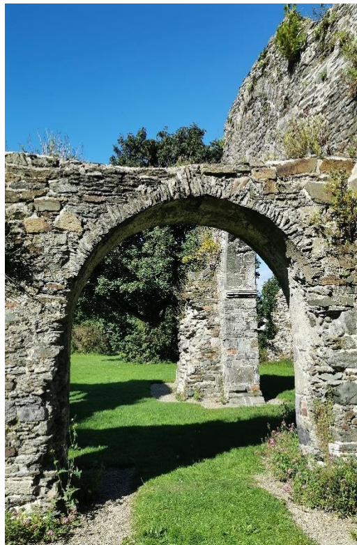
Photograph 4: Northern of two arches with misshaped barrel
