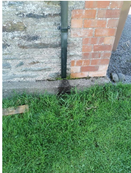
Photograph 28: Rainwater pipe missing end piece and allowing water to exist directly onto plinth to North elevation of coach house
