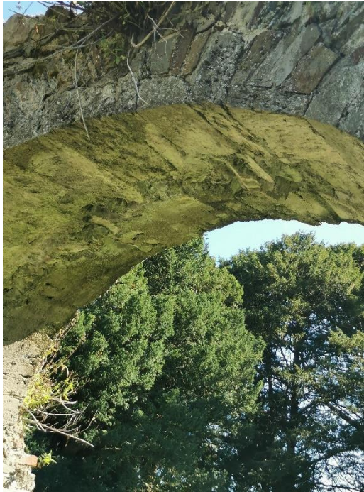
Photograph 5: Loose stones to underside of arch
