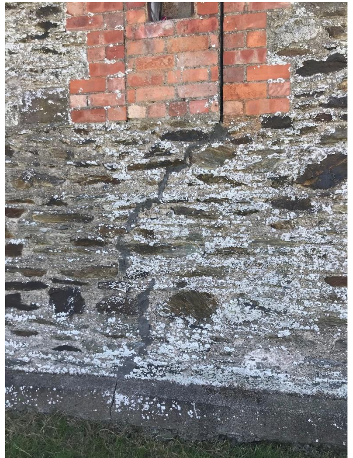
Photograph 24: Cracking in north elevation to coach house
