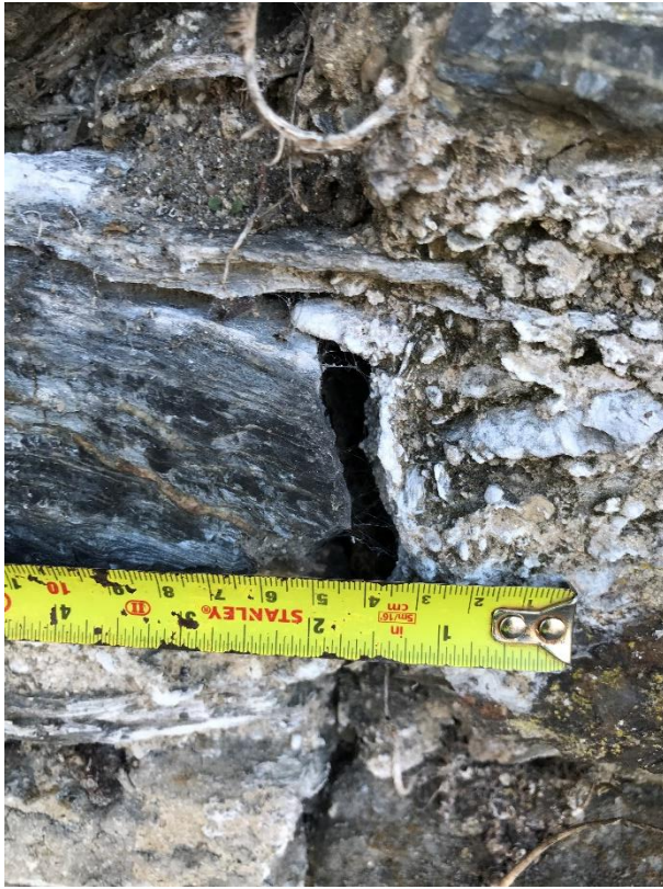
Photograph 41: Crack close up
