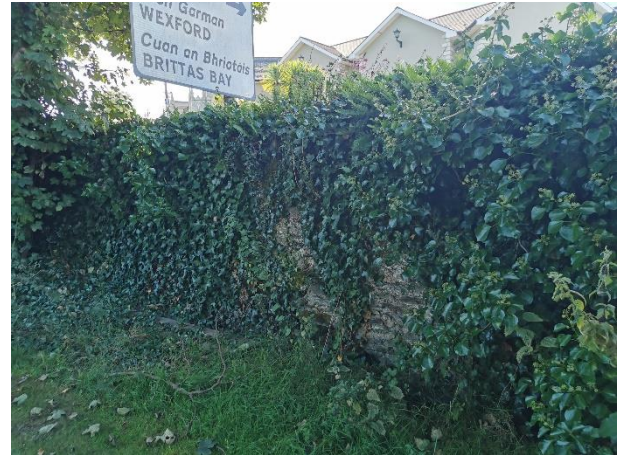
Photograph 34: Vegetation growth on boundary wall
