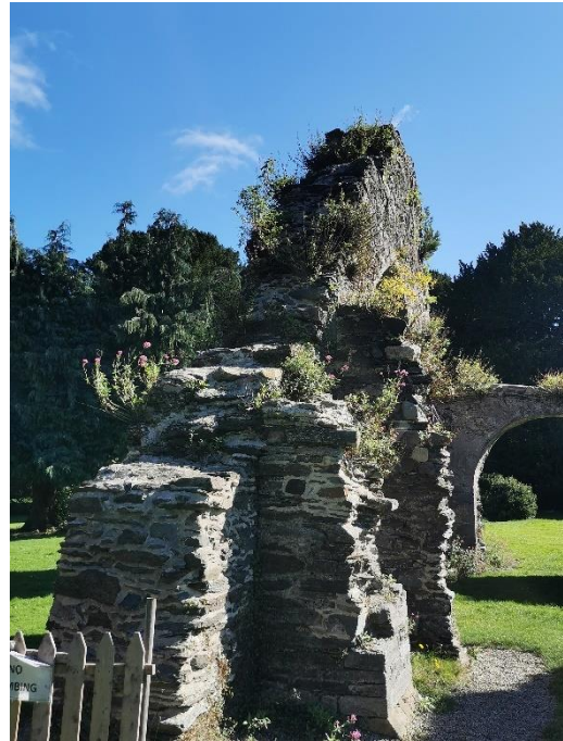
Photograph 6: Mid wall running east to west showing vegetation growth
