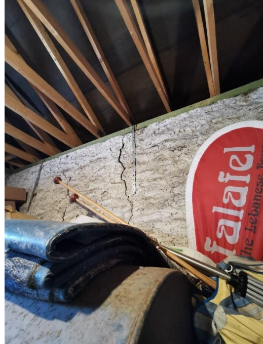
Photograph 14: Cracking to inside face of wall
