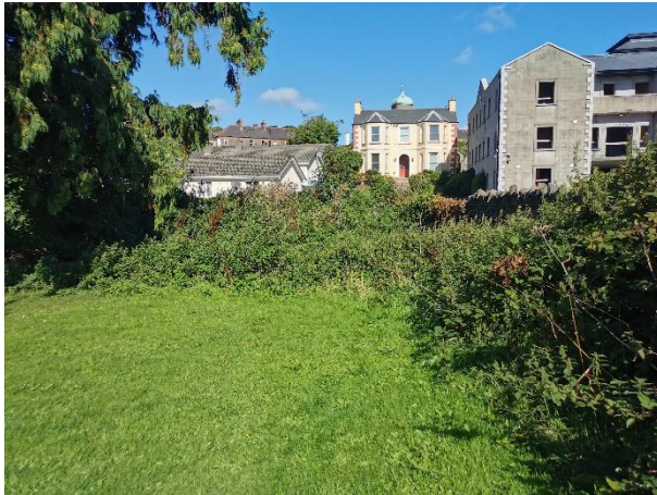
Photograph 33: Overgrown vegetation to boundary wall
